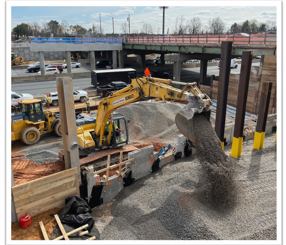
An excavator shovels gravel into the western abutment of the new Georgetown Pike bridge (March 2024)
