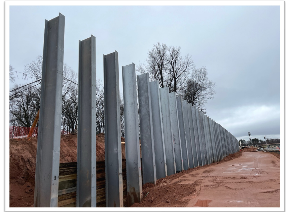
More than 90 noise wall posts installed along northbound I-495 between Georgetown Pike and Live Oak Drive (March 2024)
