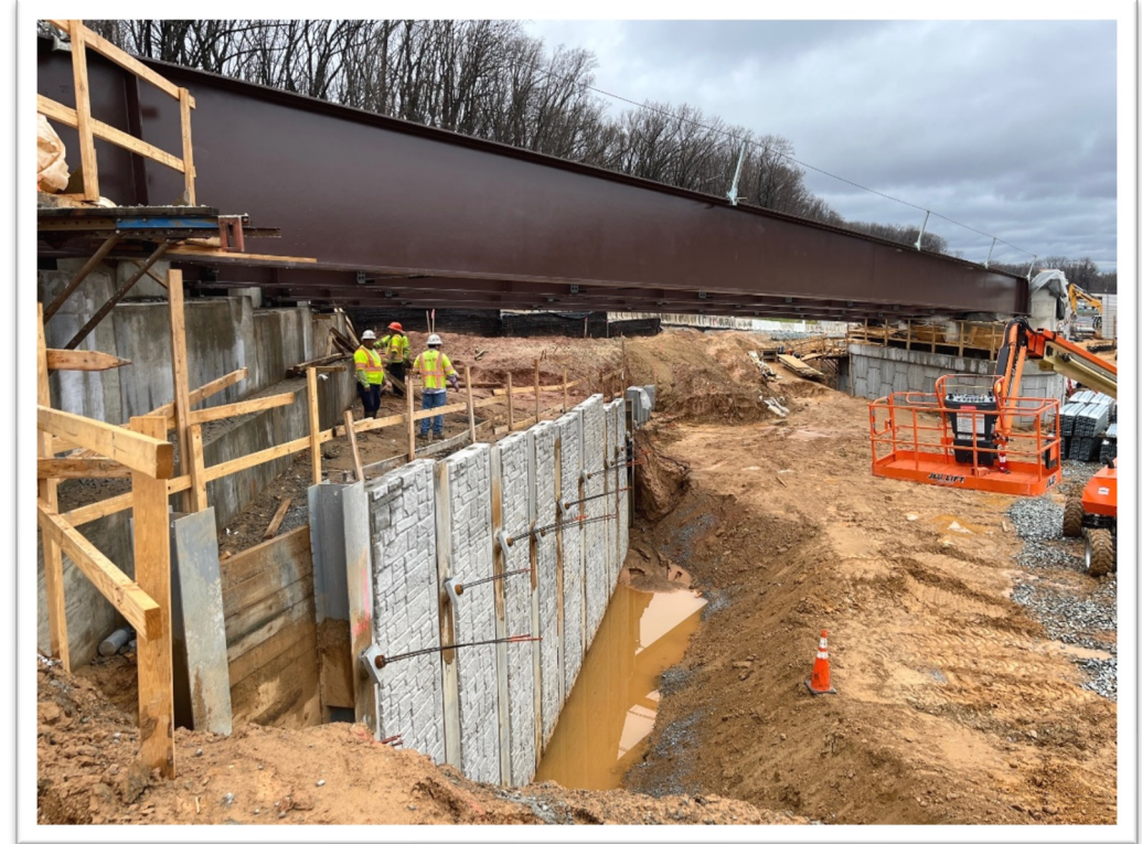
Four 100-ton girders were lifted into place for an overpass for the future southbound I-495 to Georgetown Pike ramp (February 2024)
