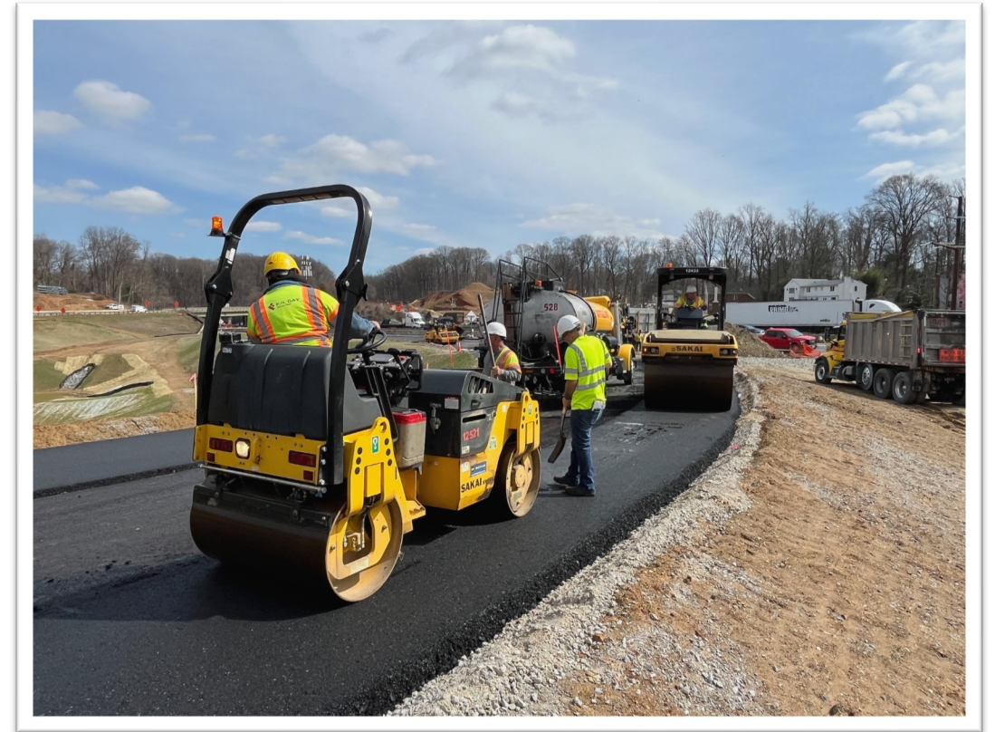
Rollers complete paving for the future GW Parkway to southbound I-495 ramp (March 2024)
