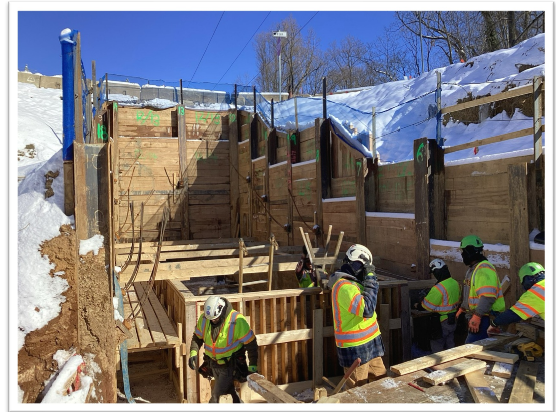
A crew works on the eastern abutment of the new Live Oak Drive bridge (January 2024)
