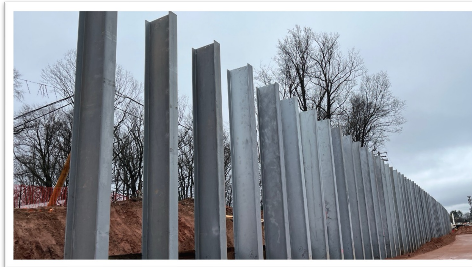
Bottom Image: More than 90 noise wall posts installed along northbound I-495 between Georgetown Pike and Live Oak Drive (March 2024)
