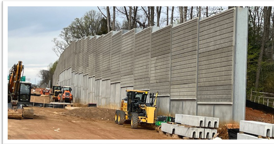
Top Image: New noise wall along northbound I-495 between Old Dominion Drive and Georgetown Pike (March 2024)
