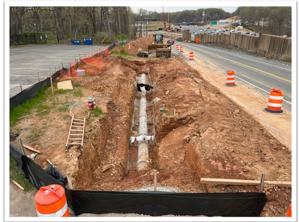
A newly completed water line adjacent to the Langley Swim & Tennis Club awaits earthen fill. (March 2024)
