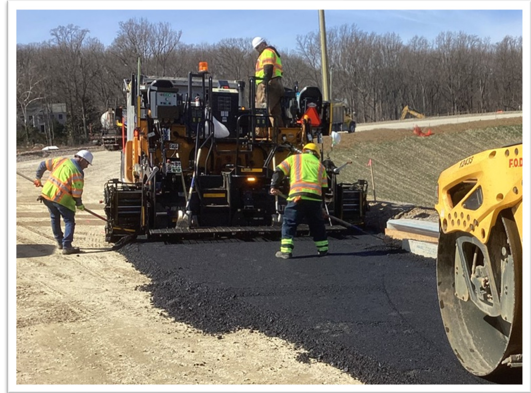
A crew lays down base asphalt for the future GW Parkway to southbound I-495 ramp (March 2024)
