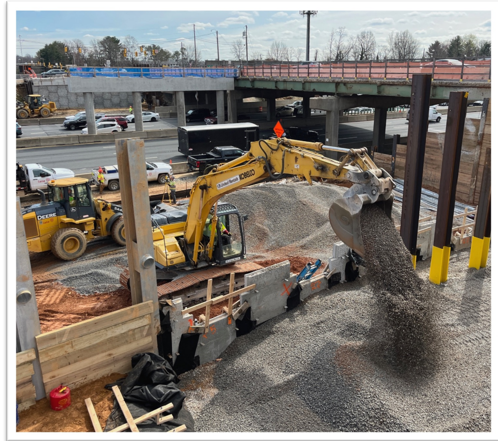
An excavator shovels crushed stone behind a retaining wall next to the western abutment of the new Georgetown Pike bridge (March 2024)
