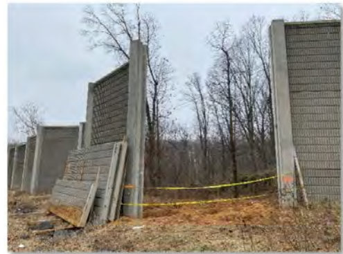
Noise wall panels removed to provide access for boring rigs along southbound I-495 between Georgetown Pike and Old Dominion Drive.
